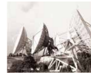
通信设备 Communication Equipment
